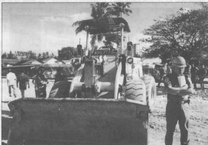
Bulldozer, enforcement officers, KTM officials and the police getting ready for demolition work.
